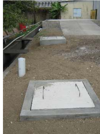
Over 600 gallons of oily waste have been pumped since March 2011
